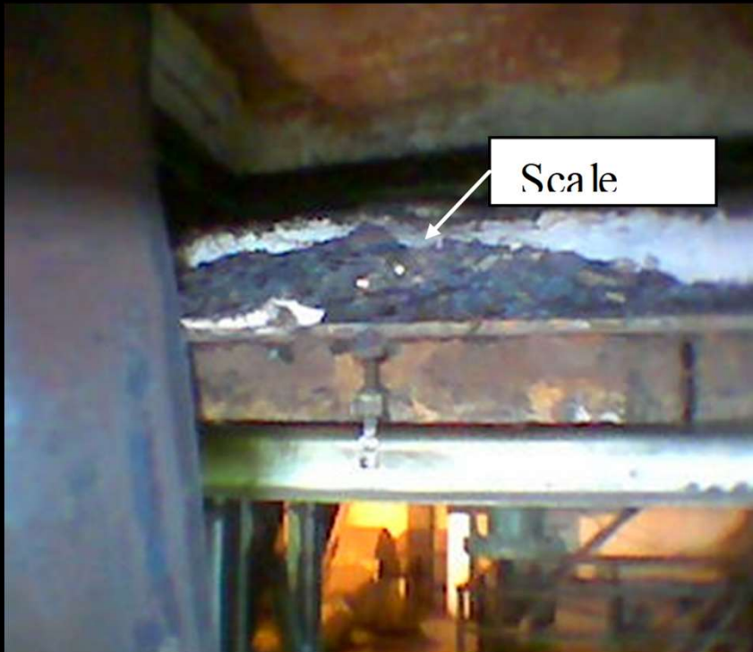
Accumulated scale at furnace bottom
