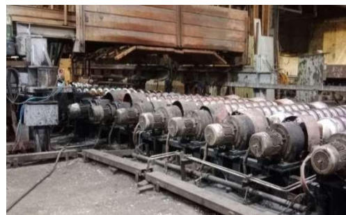
Figure 11: LASER Sensor based Slab Zero Positioning System for TCM-2 of Slab Caster-6
