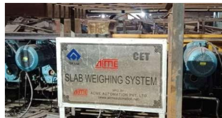
Figure 8: Slab Weighing Machine Installed at Plate Mill
