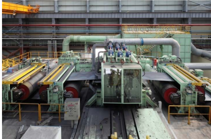
Fig 4 View of a DWU Scale Breaker
