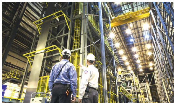
Fig 13 The ultra-high-strength steels produced in the PRO-TEC annealing line are mainly used for manufacturing crash-resistant major components in the passenger cell.
