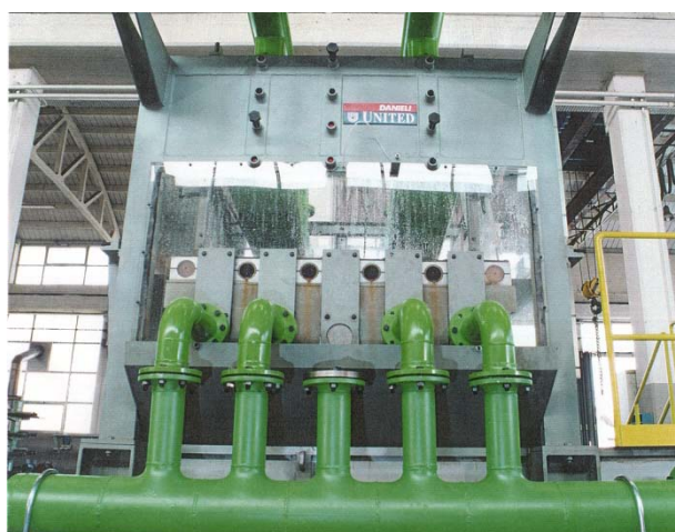
Fig 8 Intensive Cooling System
