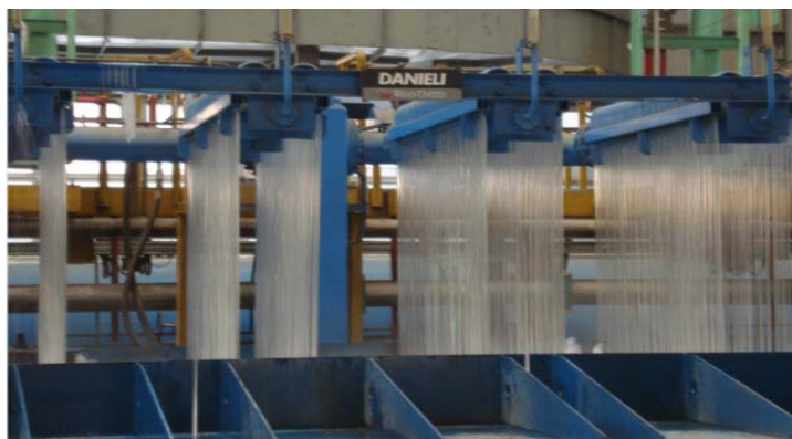
Fig 7 Specialized U-tubes type Strip Cooling Solution
