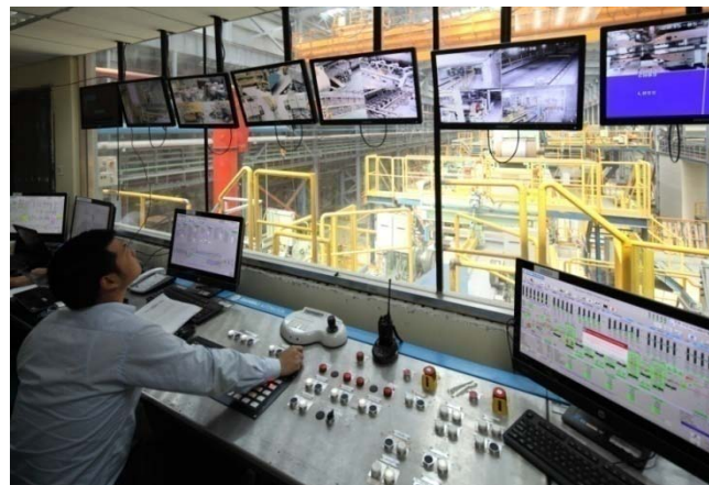
Fig.12: A view of the Control Pulpit - Danieli Automation
