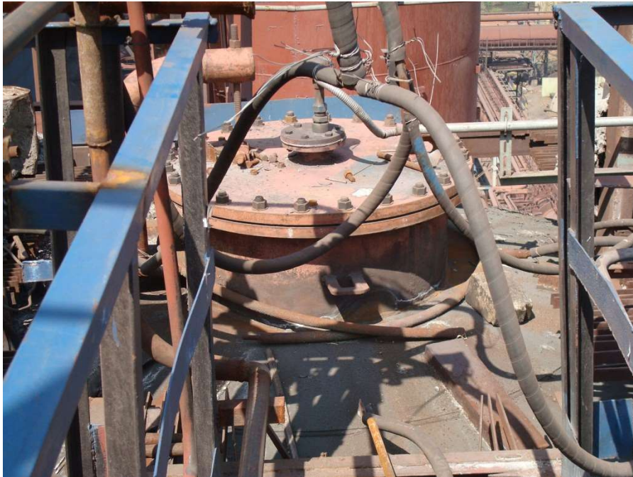
Leaking dome flange
