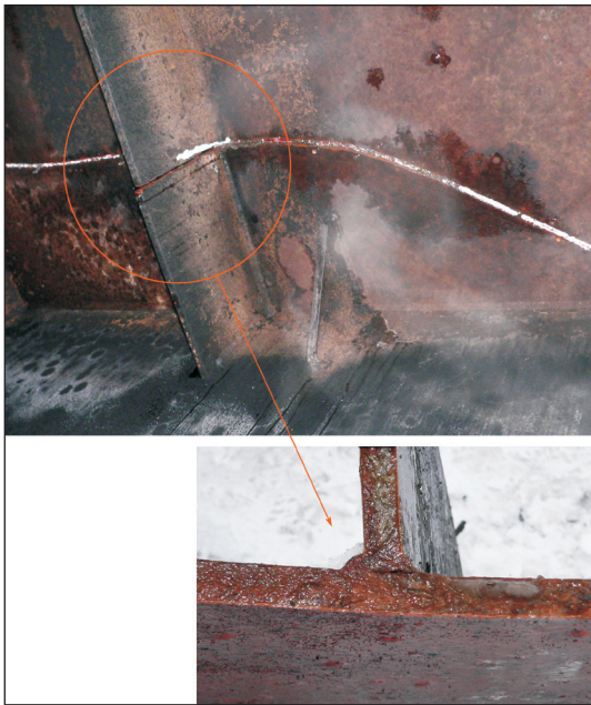
Fig. 3 : Photograph showing the crack arrest of a structure.
