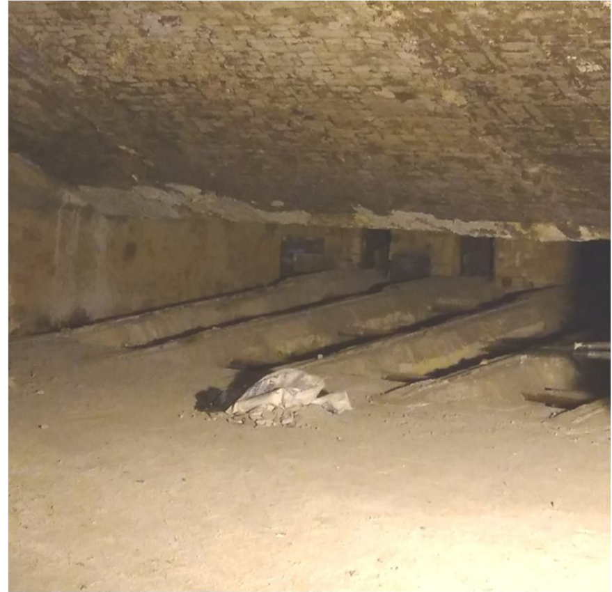
Preheating zone hearth lined with developed bricks
