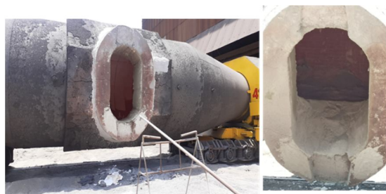
Fig.13: Condition of torpedo spout after preheating
