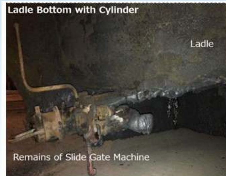
Fig 5: SN mechanism condition after Leakage between UN & UP
