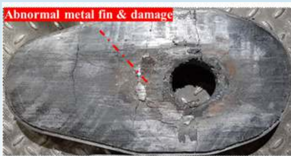
Fig 12: Slide plate stroke path damaged and metal fin observed
