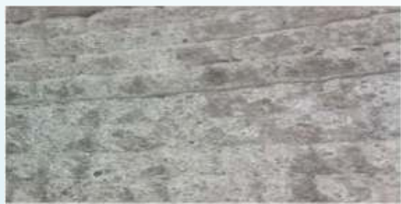
Fig-6 Ladle condition during Campaign
